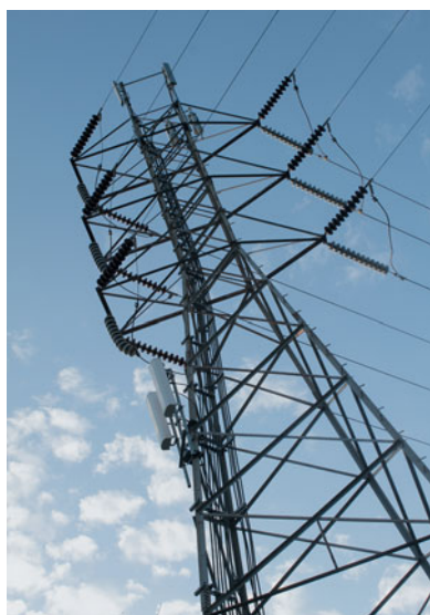
The power lines run tangent to the tower brackets at the turn.
